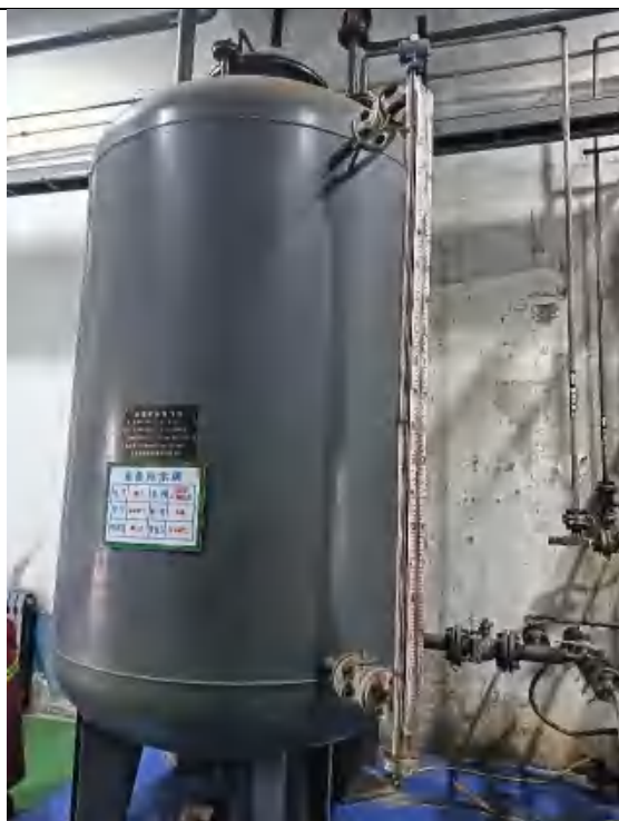
硝基苯焦油废液罐
